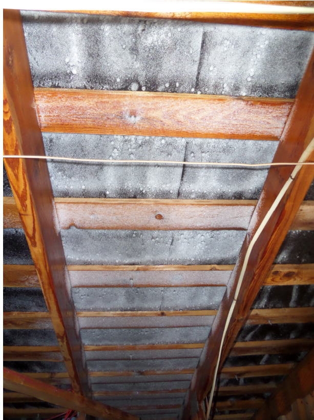
Figure 1 - Condensation near gable end of structure.
