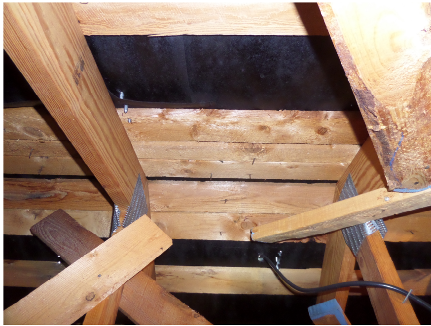
Figure 2 - Apparent obstruction of ridge vent.
