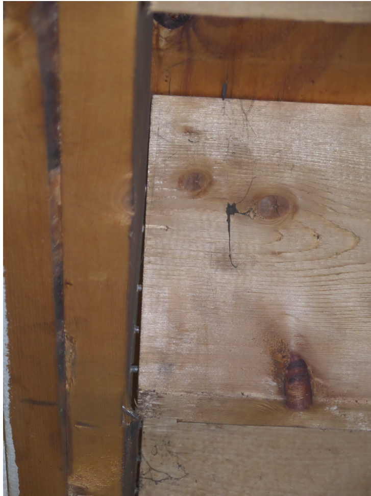
Figure 6 - Office floor joist end separating from header.
