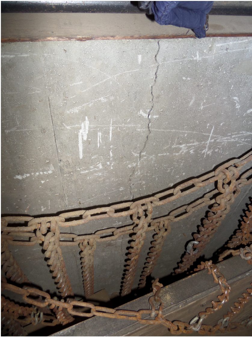
Figure 5 – Crack in concrete foundation wall.
